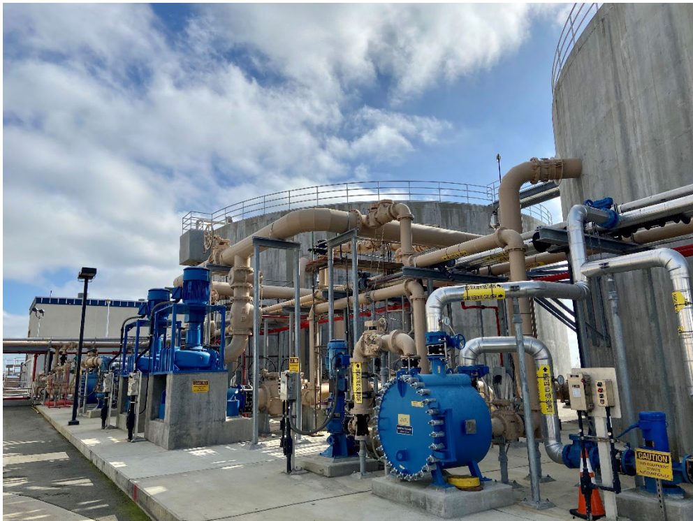
Castro Valley/Oro Loma Wastewater Treatment Plant
